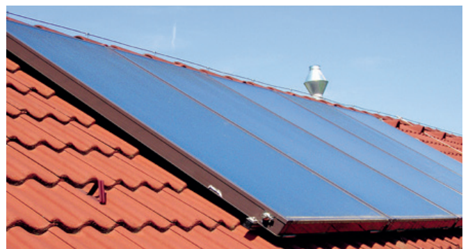
4 Solar thermal panels
