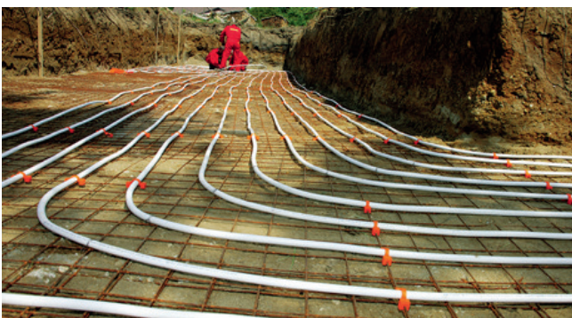
3 Underground thermal energy storage unit
